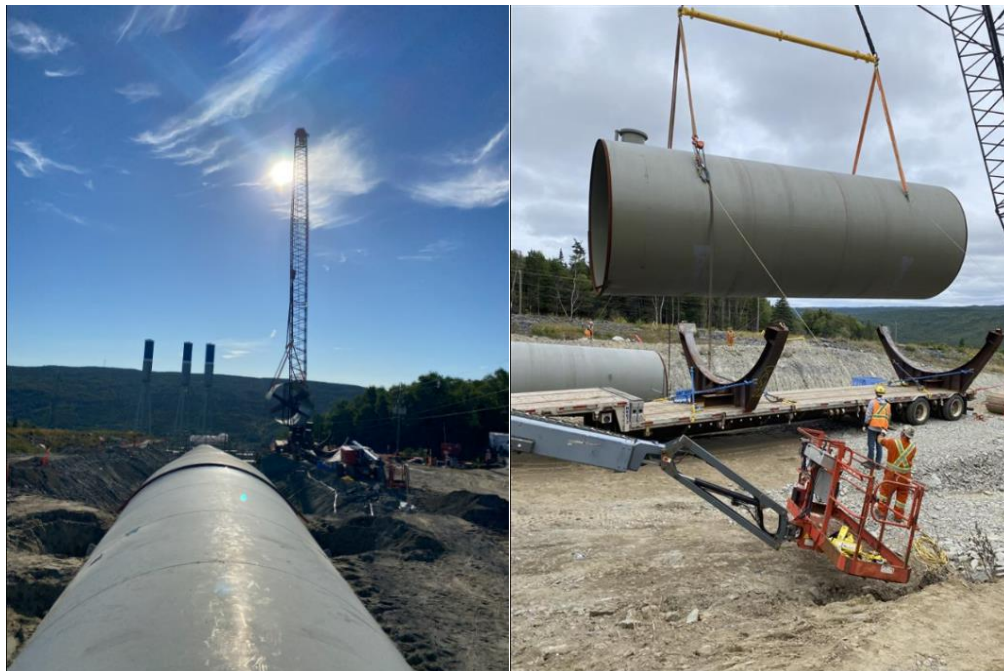
Figure 1: Placement of Can 21 and 22
